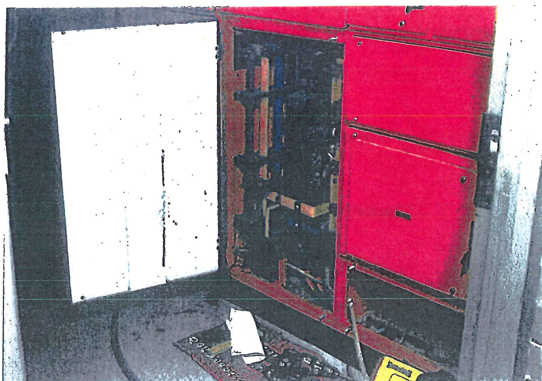
Photo 1. This image is of the view of Switch room looking from east door.
